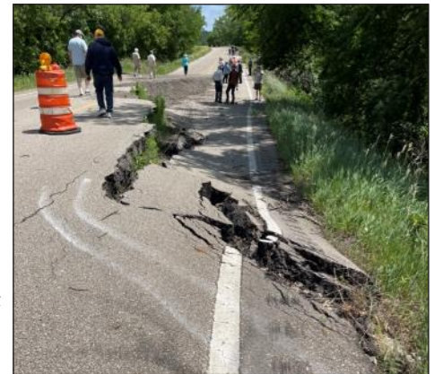
The road is unstable due to slow motion movement of the earth under the roadway
